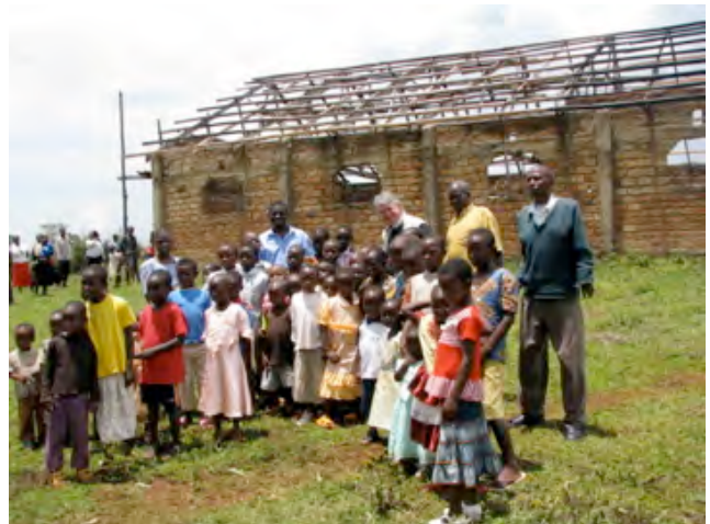
Children from the congregation of Kerino, south of Itierio, southwest Kenya, in April. The church's roof has recently been completed.
