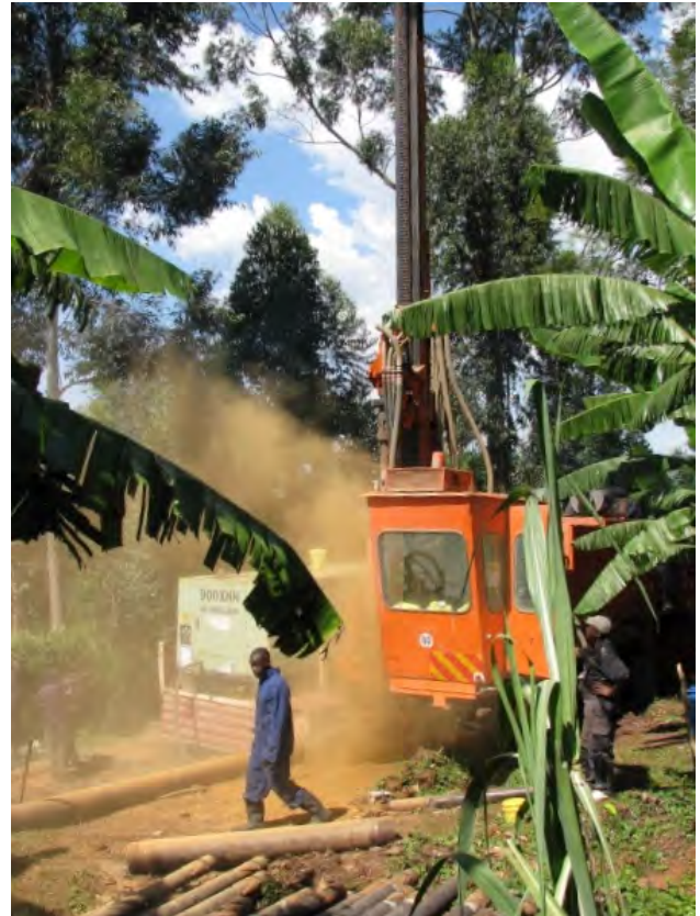
Red orange dust from volcanic soil and rock flies upward as drilling commences on the new bore hole, overseen by a hydrologist from Kericho, November 22, 2010. The well will supply the college as well as community with fresh, cool and drinkable water from a depth of 175 meters!
